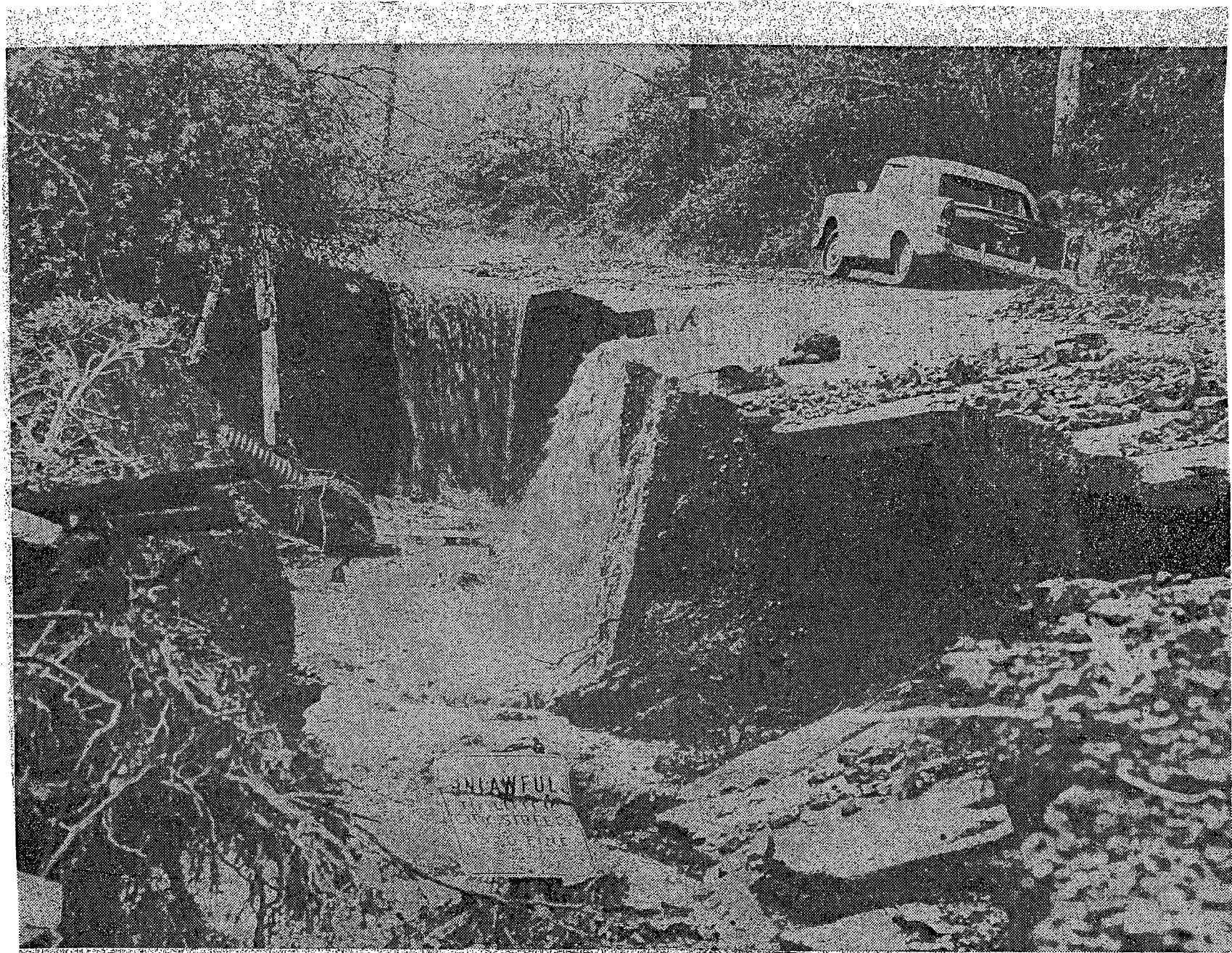
FLOOD'S POWER —Gaping hole creates a waterfall in the 3000 block of Mandeville Canyon Road—one of many washouts in the area. Times photo by Frank Q. Brown
