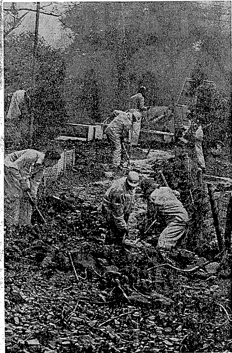
REMOVING A 'PLUG'—Maintenance crewmen work to open drainage in rock-filled ditch paralleling Mandeville Canyon Road.
